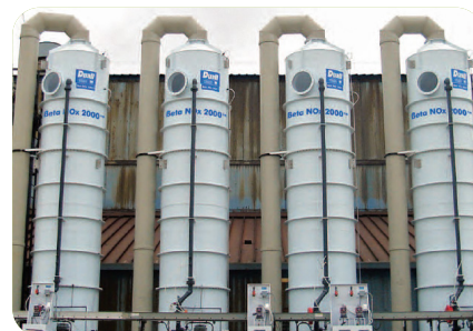
NO x Scrubber
