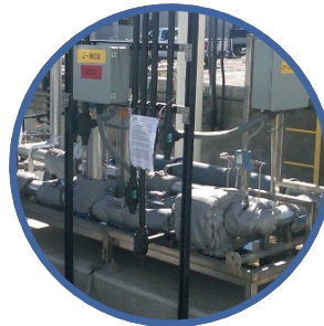
Urea or Ammonia Pump Skid
