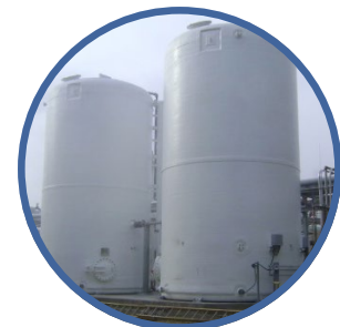
Reagent Storage Tank
