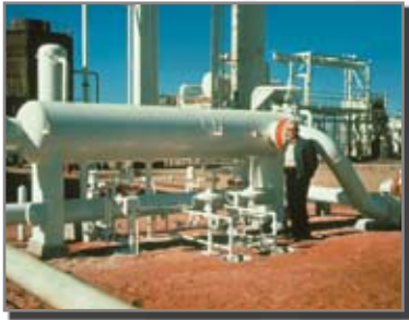
PEERLESS DOUBLE-BARREL SLUG-CATCHERS EFFICIENTLY REMOVE BULK LIQUIDS FROM HIGH GAS FLOWS.
