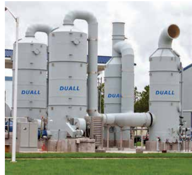
DUALLast® Degasifiers, Scrubbers, Fans, and Stacks
