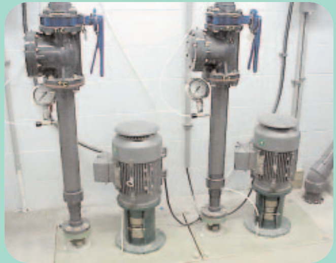
Fybroc Series 5500 Vertical pump installation
