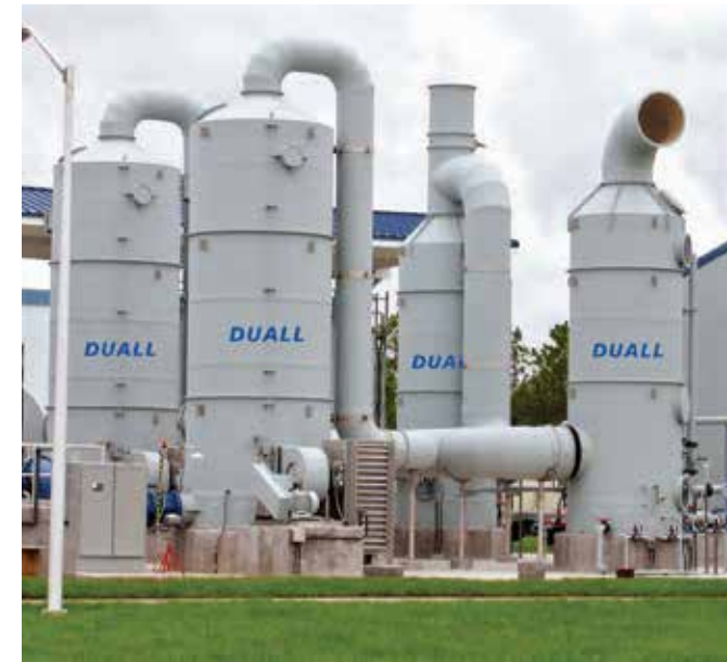
DUALLast® Degasifiers, Scrubbers, Fans, and Stacks
