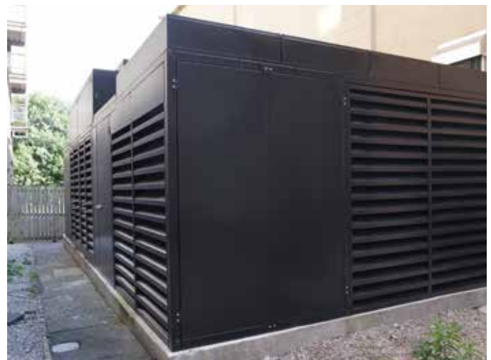
Bespoke acoustic enclosures for chillers and condensing units.
