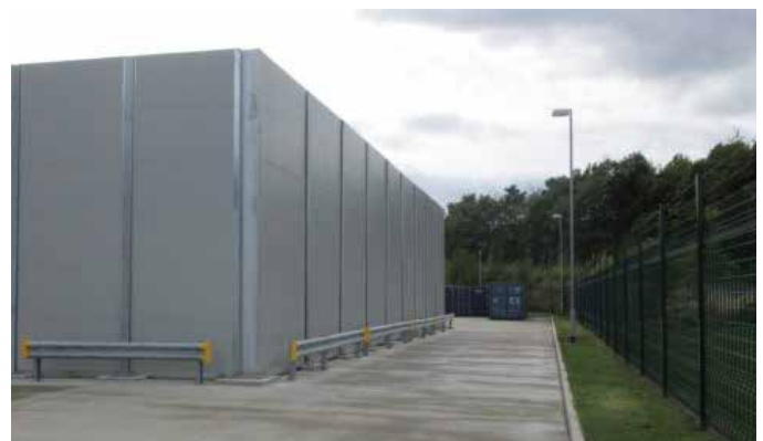
Acoustic screen and structural steelwork supports for external plant compounds.
