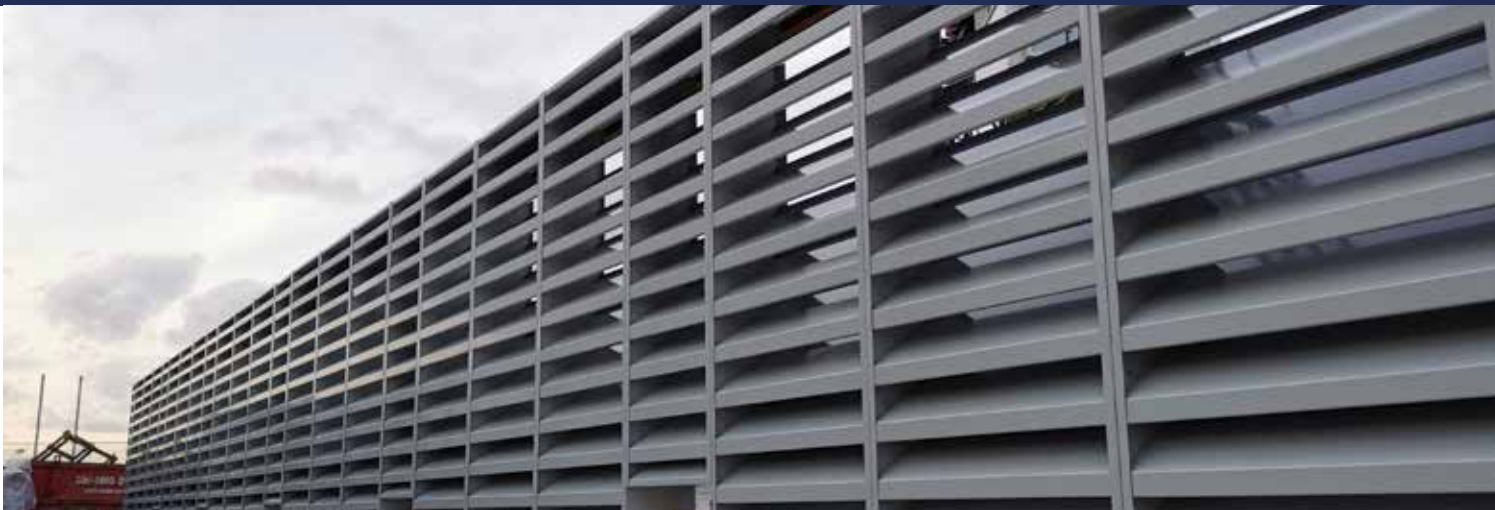
Acoustic louvred screens to roof top plant compounds.
