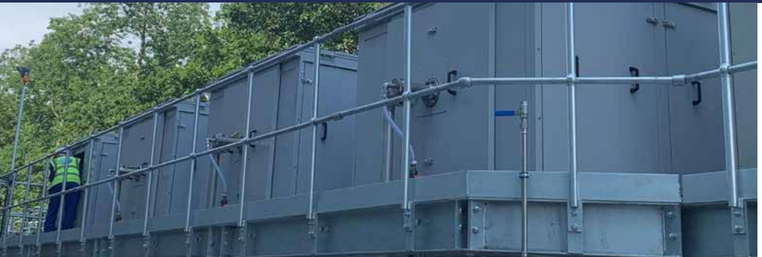
Enclosures for processing plant.
