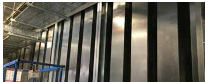
Plantroom ventilation for power generation plant.
