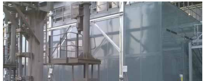
Bespoke site built enclosures for electrical transformers.
