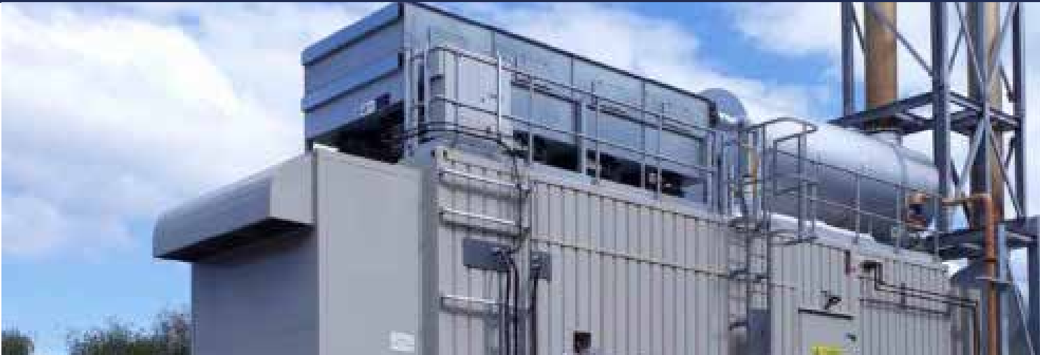
Acoustic containers for gas and standby diesel power generation plant, and CHP systems.
