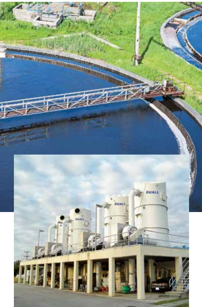
Water Production Plant with Degasifiers
