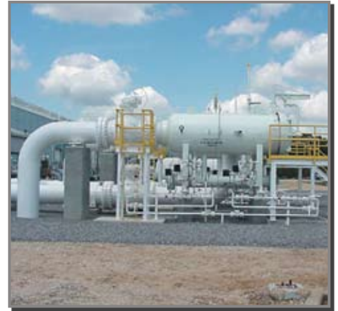
THIS PEERLESS FILTER-SEPARATOR IS INSTALLED AT A COMPRESSOR STATION IN NATURAL GAS TRANSMISSION SERVICE. THIS PEERLESS UNIT IS DESIGNED WITH A COST-EFFECTIVE FULL-DIAMETER CLOSURE.
