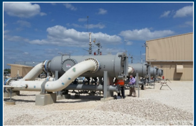
ULTRA filter-separators installed in parallel for final cleaning of natural gas before liquefaction.
