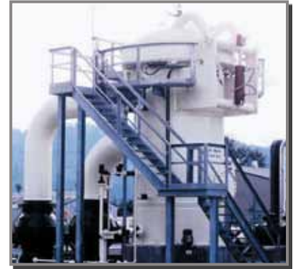
THIS ABSOLUTE SEPARATOR IS INSTALLED IN A METERING STATION IN CANADA. ITS 99" ID HOUSING UTILIZES A FULL DIAMETER, QUICK-OPENING CLOSURE.
