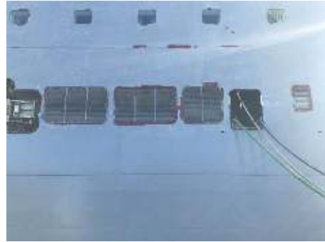
Figure 14: Tools for welding and grinding require electrical cables and pneumatic hoses to be dragged through access ports aboard USN Charles Drew (T-AKE-10)
