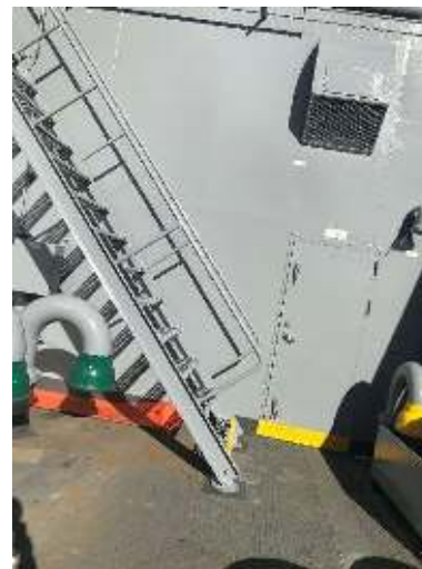
Figure 20: Freshly repaired and painted steel ladders aboard USN Charles Drew (T-AKE-10) may last for three years until the next maintenance cycle and will ultimately need to be replaced in full
