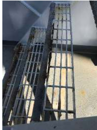
Figure 19: Steel ladder treads aboard USN Charles Drew (T-AKE-10) require periodic repair, but will ultimately need to be replaced when the base metal corrodes
