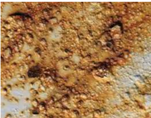
Figure 2: Close-up of a corroded steel louver blade with blistered paint
