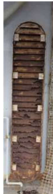
Figure 4: Shiplide louver blades experiencing severe corrosion aboard LSD-class
