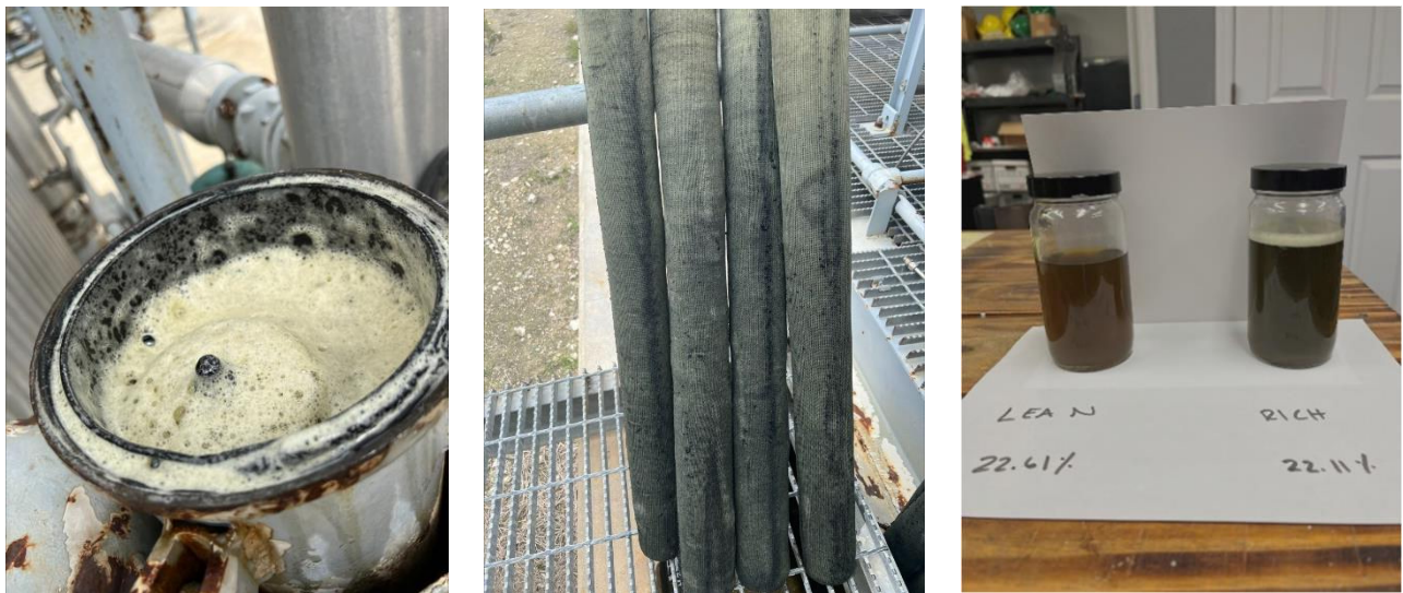
Figure 3 – Amine Foaming in Pre-Carbon Filter, Black Debris on Filter Cartridges, and Amine Samples
