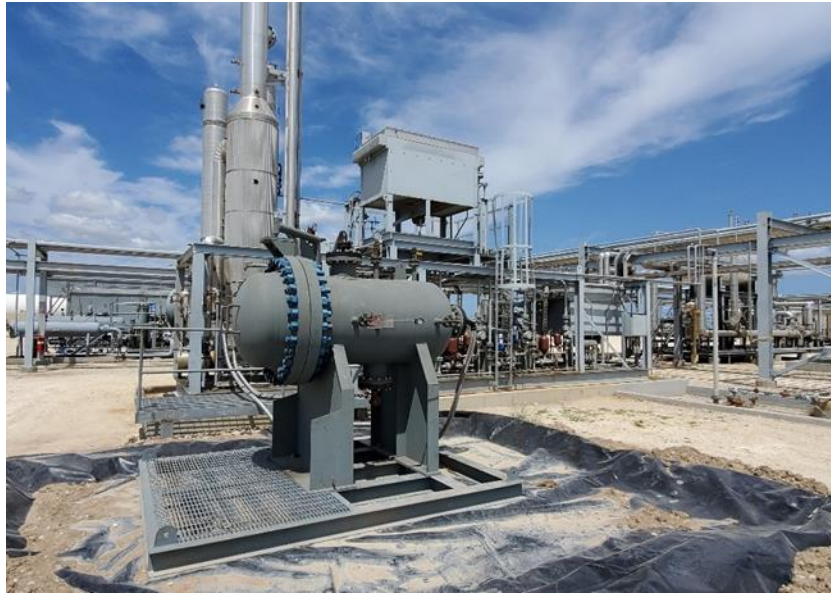
Figure 8 – Installed Rental Vessel at HEP Live Oak Facility
